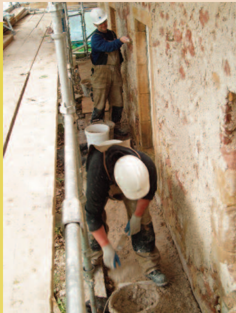
Benny and Finton are carrying out this work on the south wall
