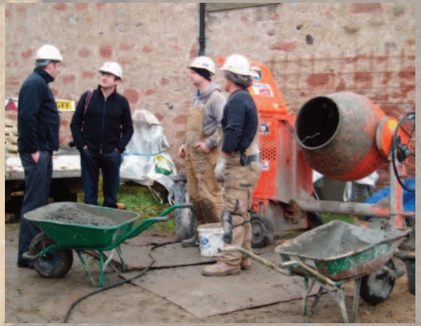
The concrete floor has been debated
